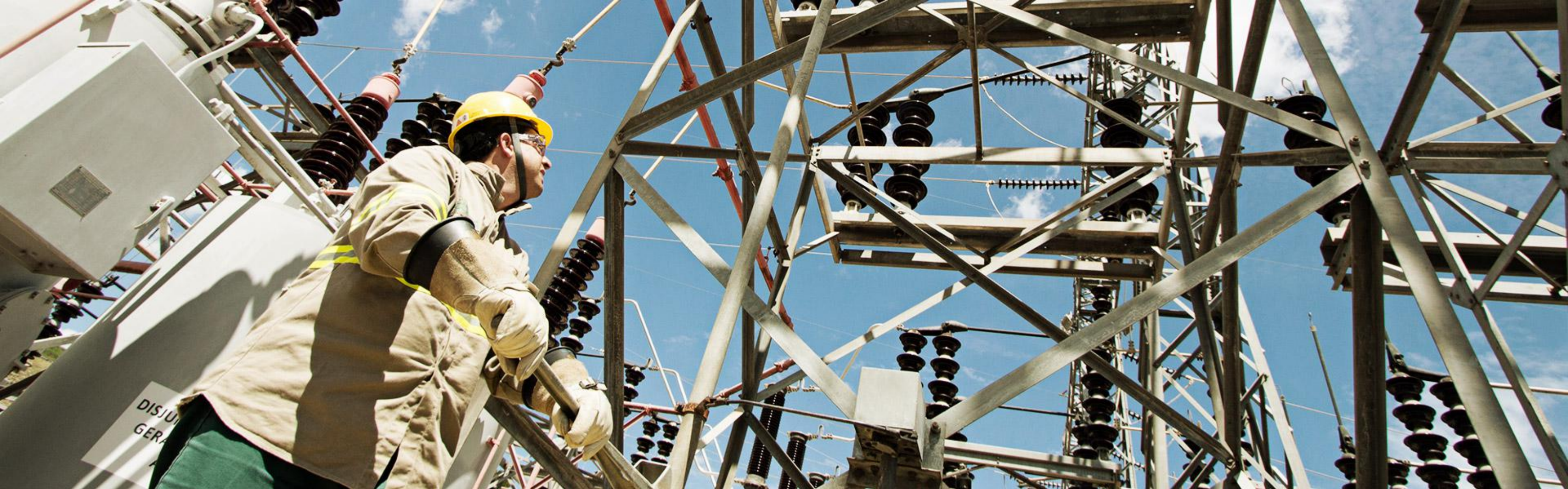
Wanderson José Rodrigues de Carvalho, plant operator, during the execution of maneuvers at the substation of the Itutinga Hydroelectric Power Plant.
