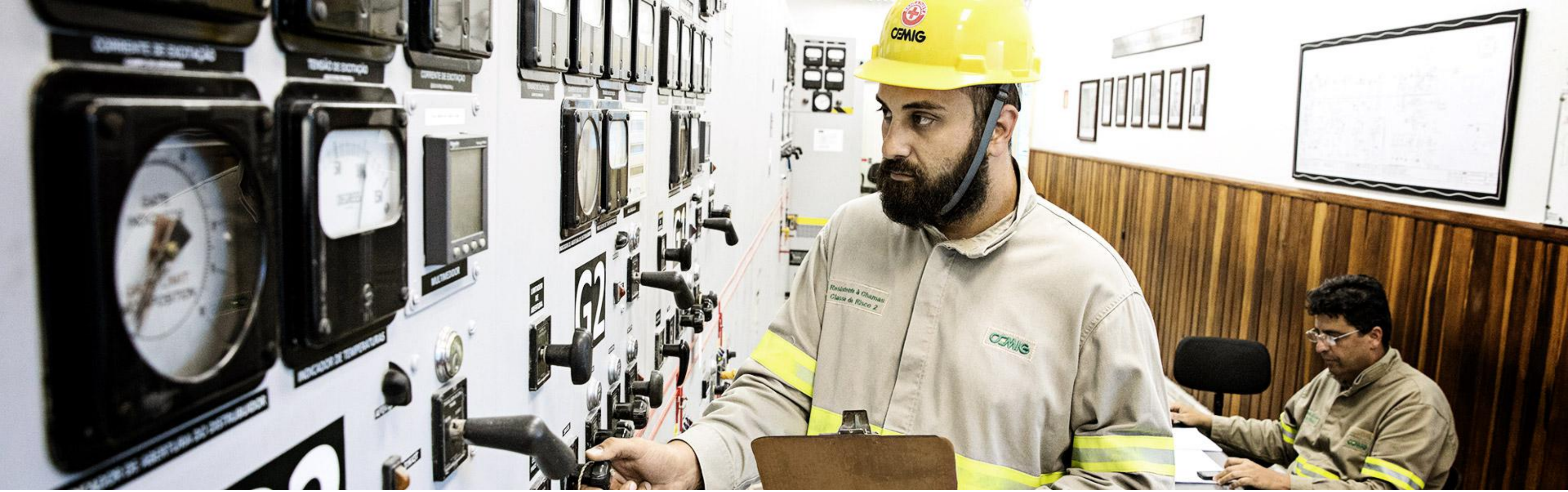
Mario Pinto, technician of operation during the accomplishment of maneuvers in the control room of the Itutinga Hydroelectric Power Plant. In the background, Wanderson, operator. Itutinga-MG, Brazil.
