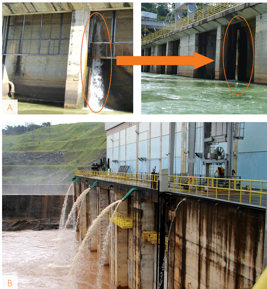
FIGURE 4 – Cooling water pipe of the Trés Marias Dam power generation units (A). Elongation of the cooling water outlets away from the powerhouse walls of Funil Dam (B).
