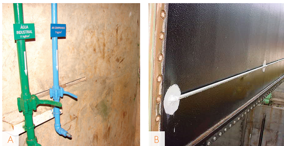
FIGURE 6 – Water (green pipe) and compressed air (blue pipe) injection pipes of Emborcação Dam (A) and an aeration system (white pipe) on the stoplog panel of Funil Dam (B).
