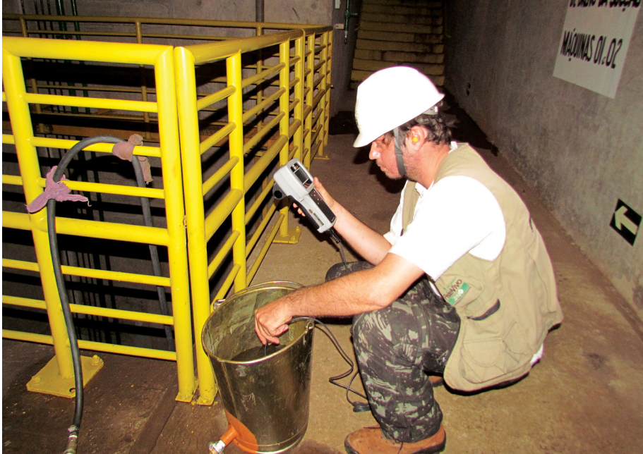
FIGURE 5 – Measuring dissolved oxygen of the draft tube water during turbine dewatering at Amador Aguiar I Dam. Photo: Átila Rodrigues Araújo.
