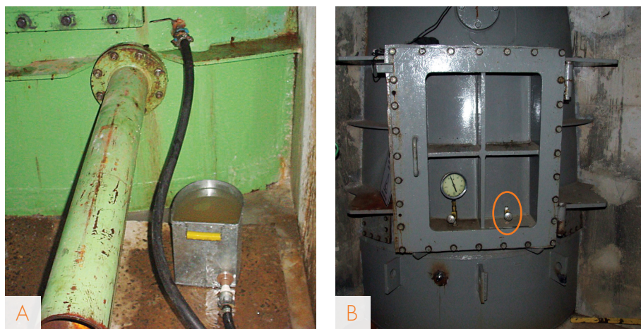
FIGURE 5 – Installation of stations for monitoring dissolved oxygen in the hatch of the draft tube at Funil Dam (A) and Rosal Dam (B).
